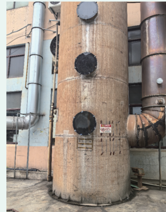
Decontamination Furnace Waste Gas Discharge Outlet Signage (Before Rectification)
