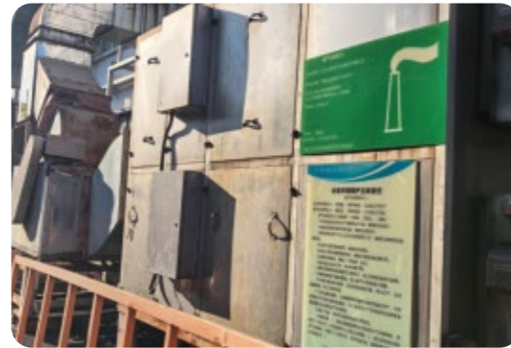
Air emissions treatment equipment
