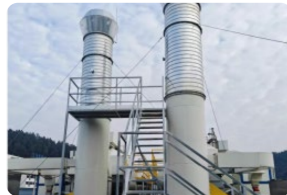
Air emissions treatment equipment
