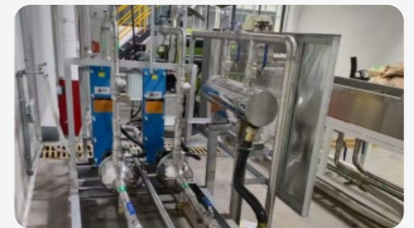
Granulation Circulating Water Cooling System
