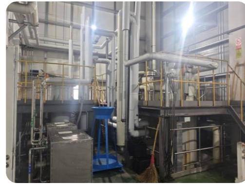
Triethylene Glycol Cleaning Equipment
