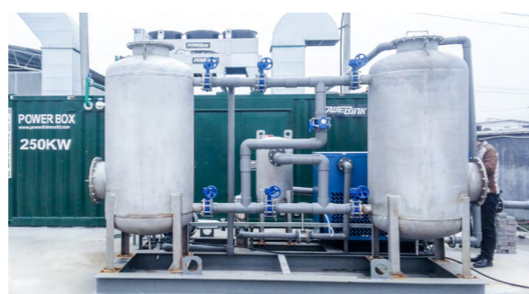
On-site biogas power generation facilities
