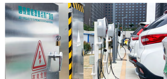
Charging piles for electric vehicles in Muyuan
