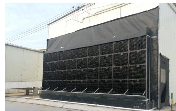
On-site deodorization and sterilization system
