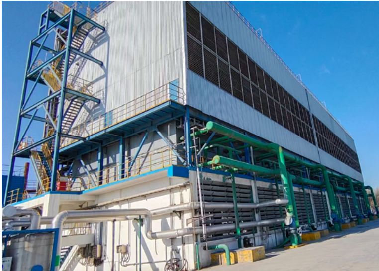
密闭循环水冷却塔干湿联合冷却塔
