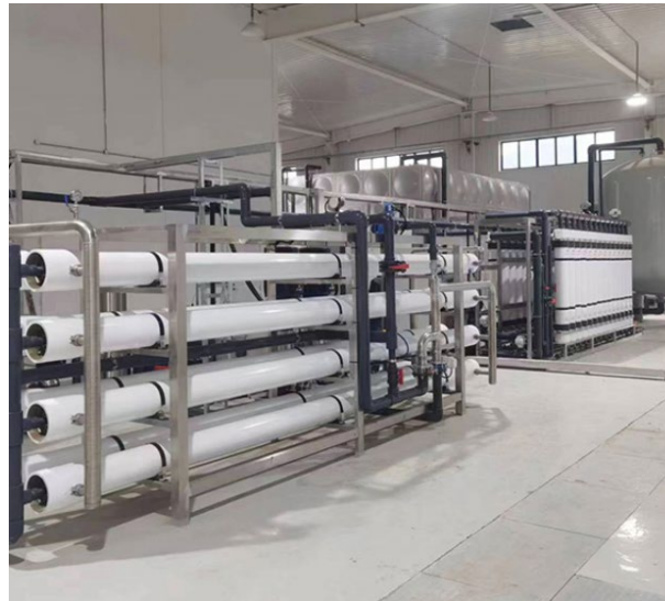
Super Factory coating wastewater treatment
