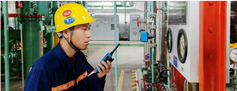
集控专业巡检人员检查运行设备状态
