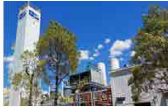
Energy-Saving Technological Transformation of On-Site Nitrogen Generation
