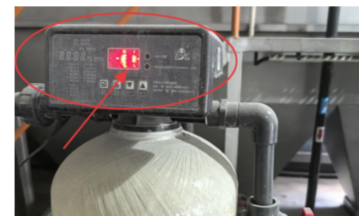
Abnormal operation of wastewater treatment sand filter
