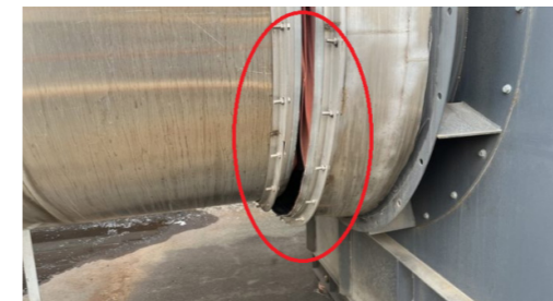
Crack in flexible pipe connection
