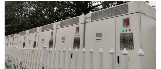
The 1 MW Energy Storage Station at the Beilun Headquarters
