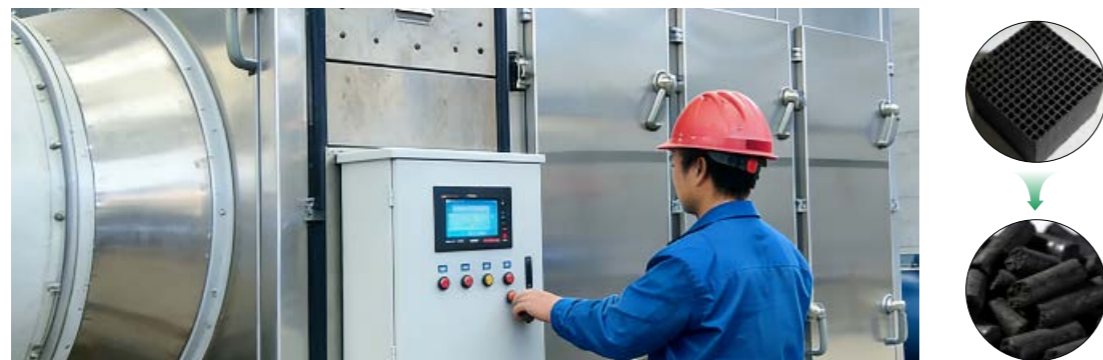
Upgraded activated carbon adsorption units to regenerable activated carbon systems
