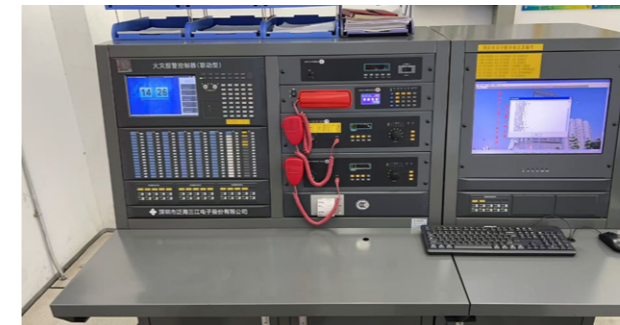
Fire Alarm Controller
