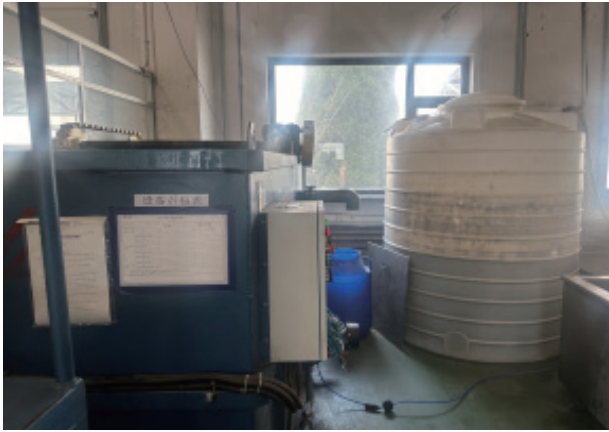
Wastewater treatment facility in the maintenance area
