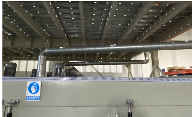
Oven in UTEC’s casting workshop connected to the waste gas disposal facility
